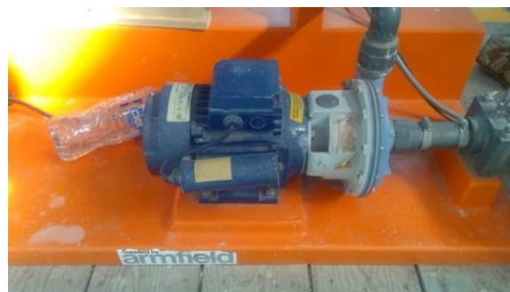
Fig. 13. Bomba Armfield Limited Ringwood Hampshire England.
